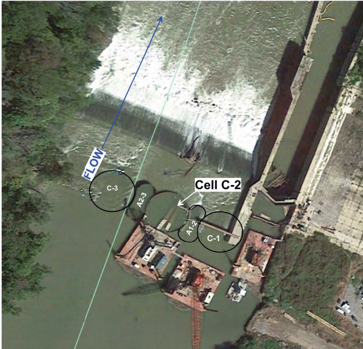
Figure 5. Location of coffer dam, Cell C-2, within the cellular dam system (September 19, 2016). The 18-m diameter coffer dam is in the process of being tremie grouted with a cement-grout mixture subsequent to the crosshole work (September 2015).
